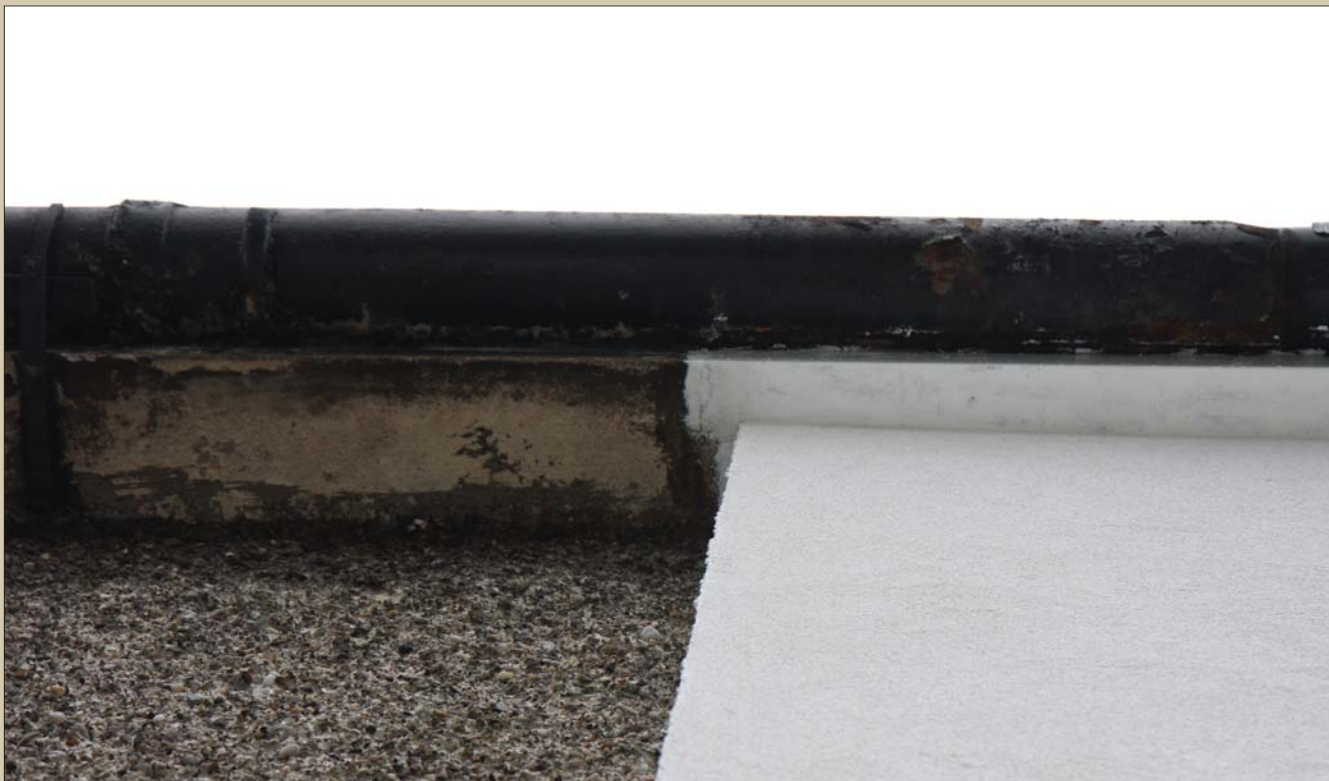
(below) 100mm of expanded polystyrene (EPS) insulation was installed externally on the front and back of the end-of-terrace house, giving the refurbished walls a U-value of 0.22 W/m 2 K. The EPS was finished externally with a fibreglass-reinforced cementitious render from Weber
